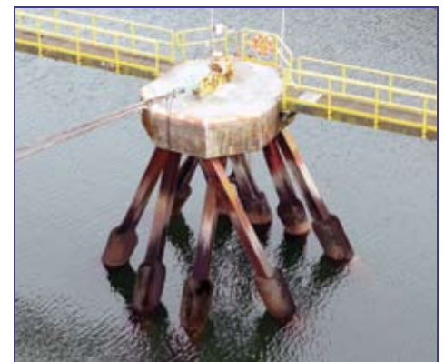
Mooring dolphins are in-water structures supported on pilings that secure vessels' lines when docked
